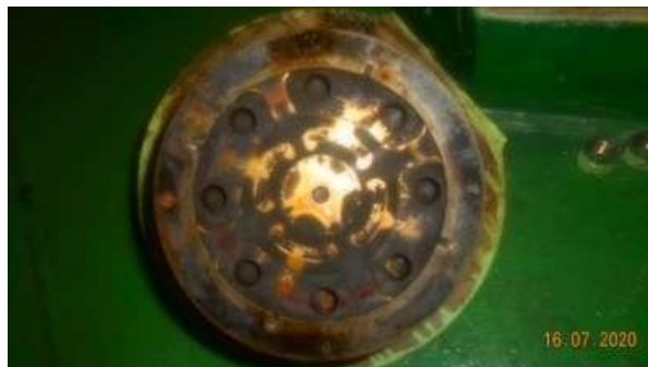
Figure 3. Low Pressure Valve
