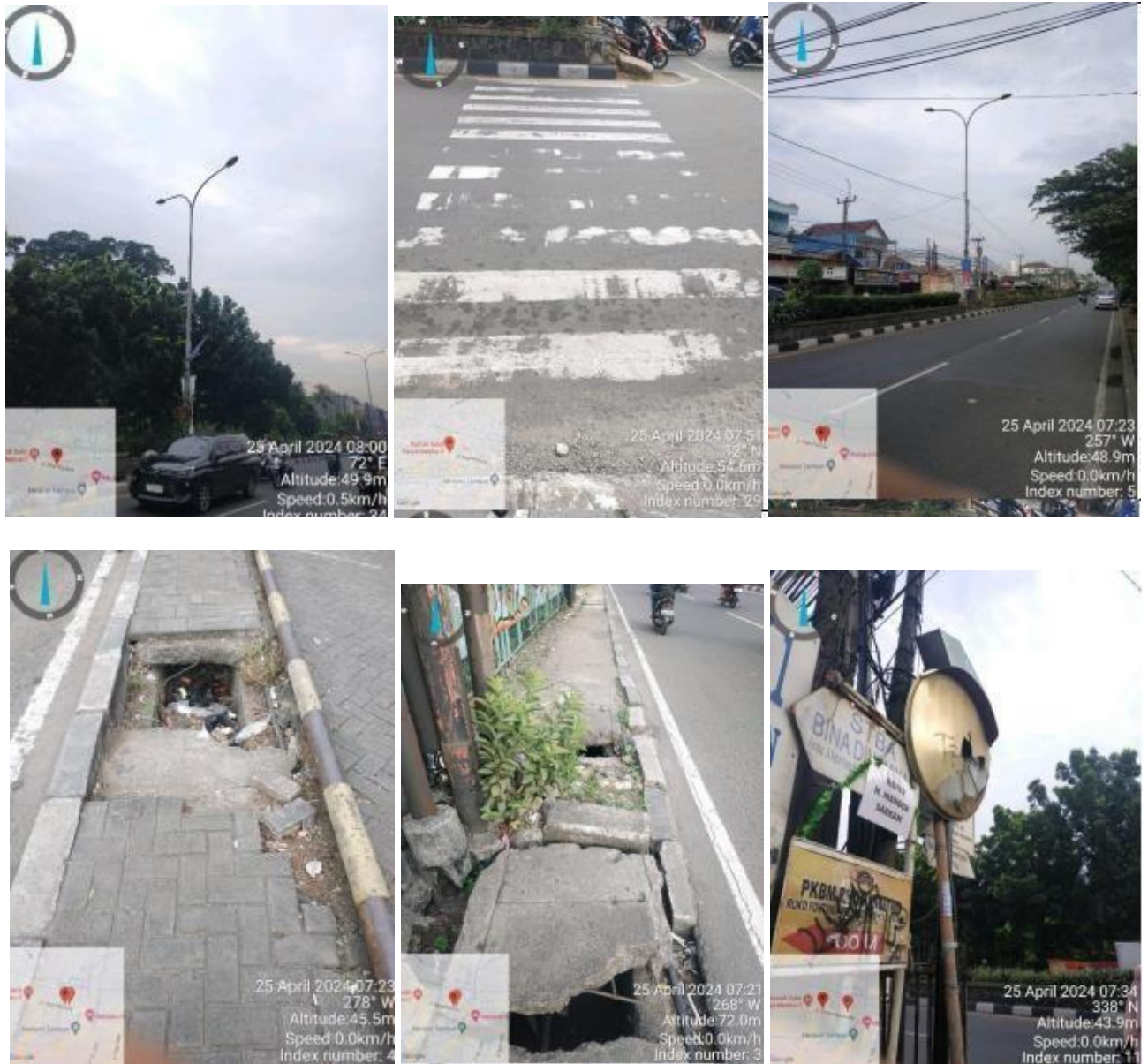
Figure 1. Condition of Study Location Jl. Teuku Umar Bekasi
